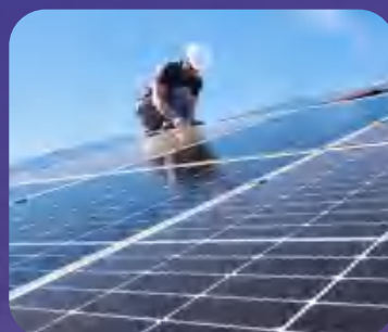
Building Photovoltaic Integration 建筑光伏一体化
